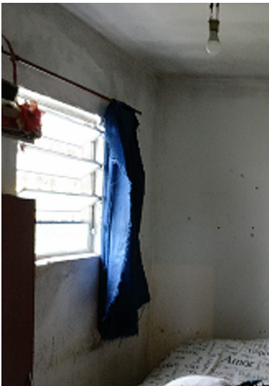
Figure 7 – House 22, undersized window for bedroom
