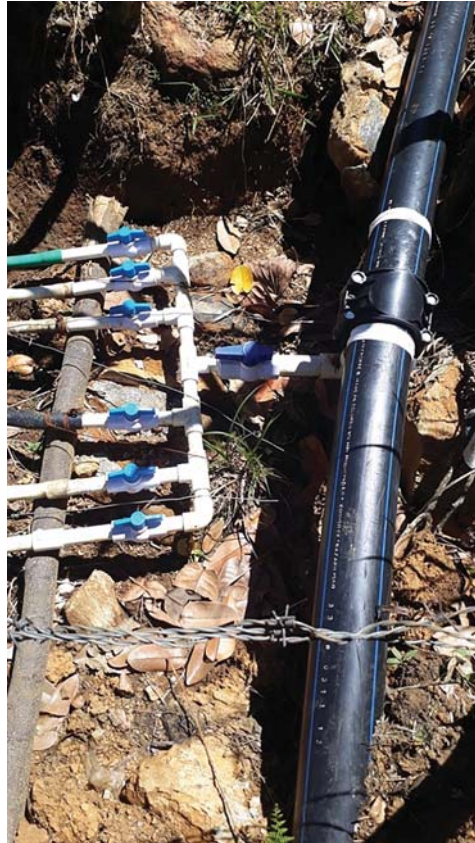
Figure 5 – Water distribution and outlet collar to “irregular” households in Bello Oriente from the communitarian pipeline
