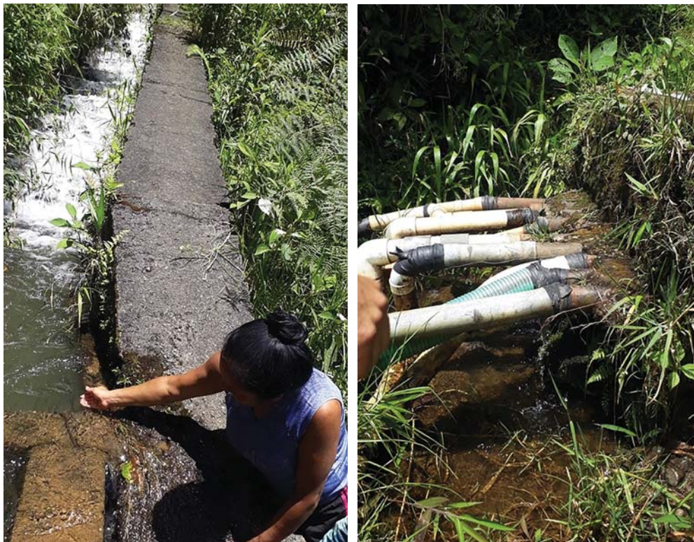
Figure 4 – EPM spillway and water collection pipes made by residents halfway down the hill
