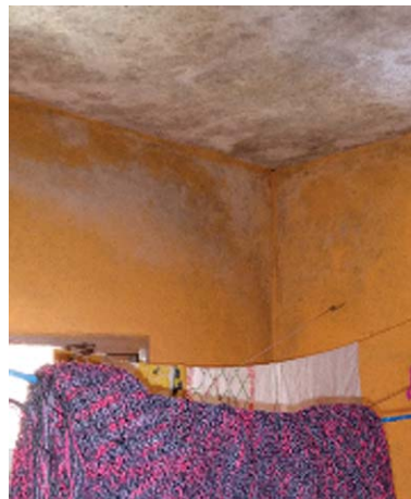
Figure 10 – House 18, mold on walls and ceiling remain even after addition of second floor
