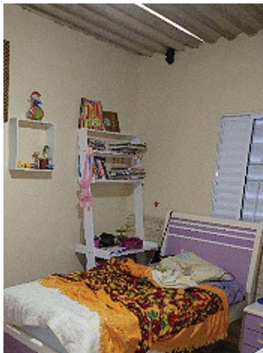
Figure 9 – House 18, visible light gap between fiber-cement sheeting after house extension
