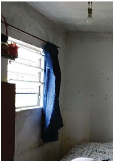
Figure 7 – House 22, undersized window for bedroom
