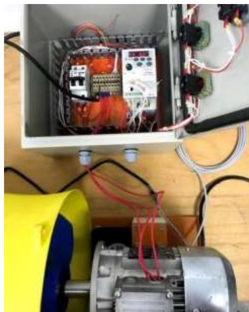
Figure 22 - Electric panel AC motor speed regulator
